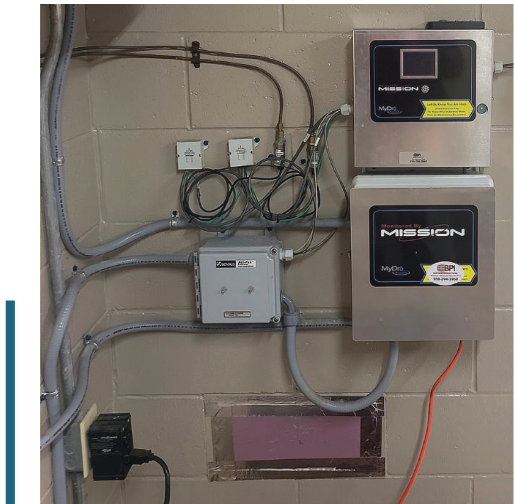
RiverSouth uses MyDro RTUs to monitor its pump station.
