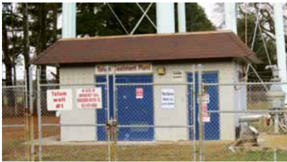
Before the new SCADA system, MWC employees made frequent visits to the Tatum (above) and McQueen (below) treatment plants to monitor the equipment.
