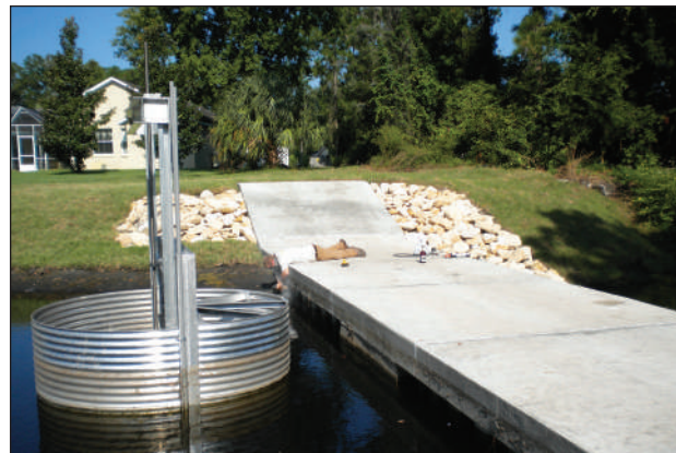
Top: The pulse inputs connected to the tipping bucket collect rainfall data, while the analog outputs control the canal gate. Bottom: Control structures with electrically actuated gates regulate flow in the canals.
